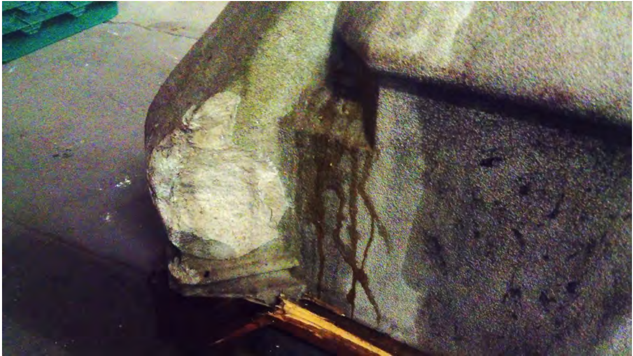
Significant loss to the stone.
